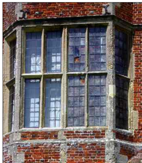
Fig. 6. The ground floor window partially bricked up on the inside. The left window is functional, but with blinds.
